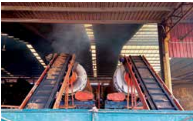
Solid Recovered Facilities in Kampung Gajah, Perak
