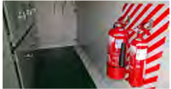
Provision of fire extinguishers in Switchgear Room at LSS2 Sik, Kedah
