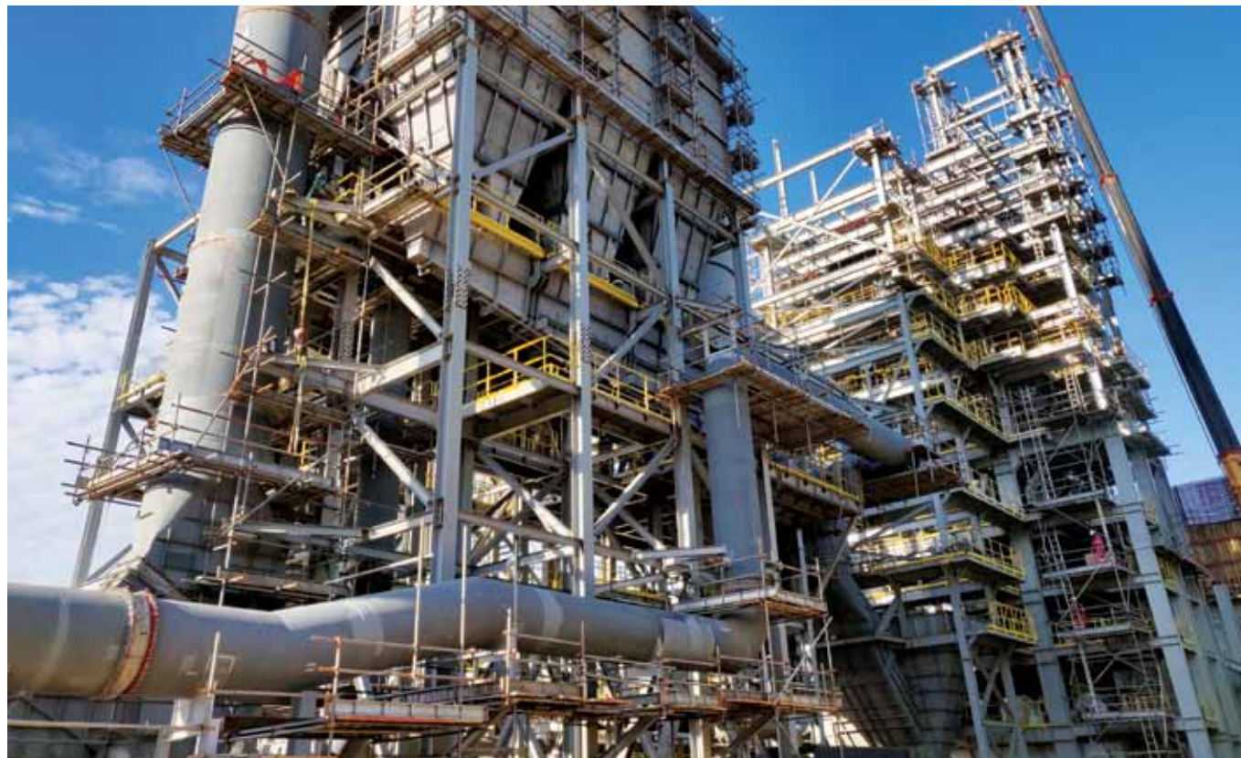
»»» View of Waste-to-Energy plant from East to West in Ladang Tanah Merah, Port Dickson, Negeri Sembilan
