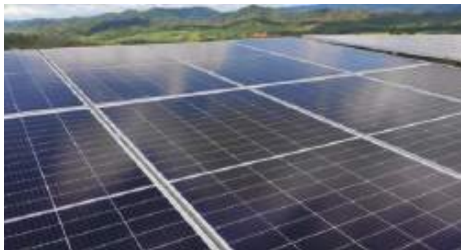
Development of Cypark's 50MWdc ground mounted solar at Sik, Kedah that worth RM 225 million.
