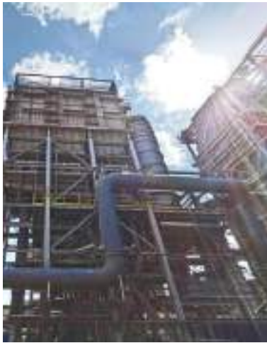
▶ Incinerator & Boiler of The SMART WTE Plant in Ladang Tanah Merah, Negeri Sembilan.
