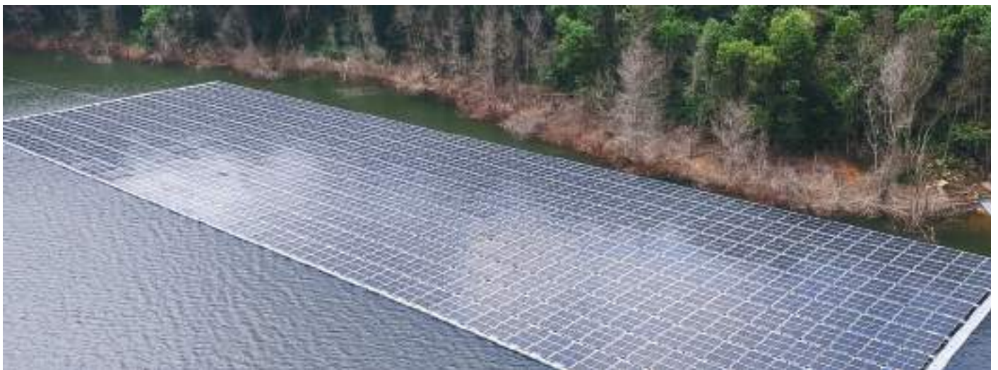
▶ Cypark is the largest EPCC for floating solar in Malaysia. Twin 100MWdc floating solar in Empangan Terip (top) and Empangan Kelinchi (bottom)
