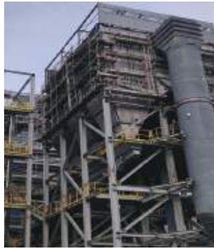
▶ Bag Filter & Fly Ash Silo of the SMART WTE Plant in Ladang Tanah Merah, Negeri Sembilan.
