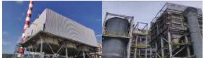
Bag Filter & Fly Ash Silo
