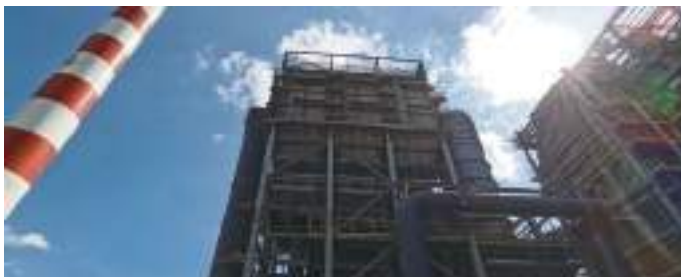
Flue Gas Treatment System & Stack
