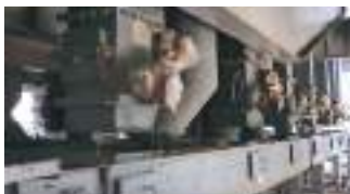
Moving Grate (External)
