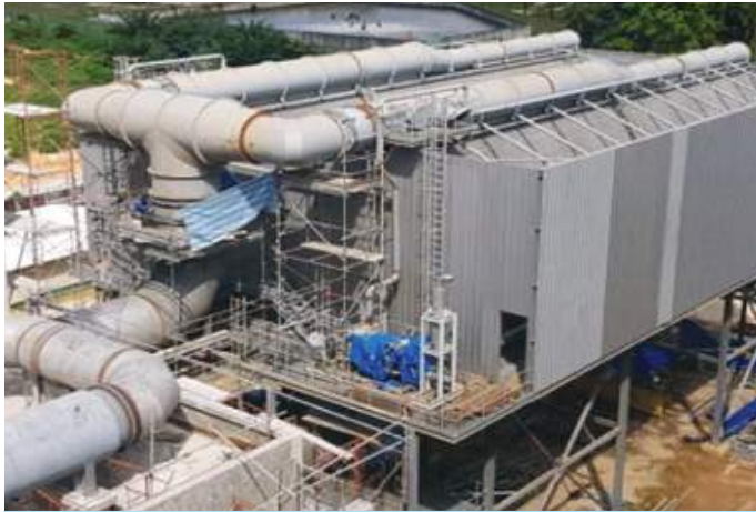
Air Cooled Condenser (ACC)
