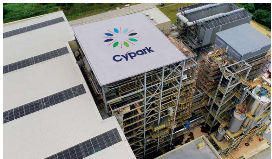
Boiler Island of SMART WTE Plant in Ladang Tanah Merah, Negeri Sembilan
